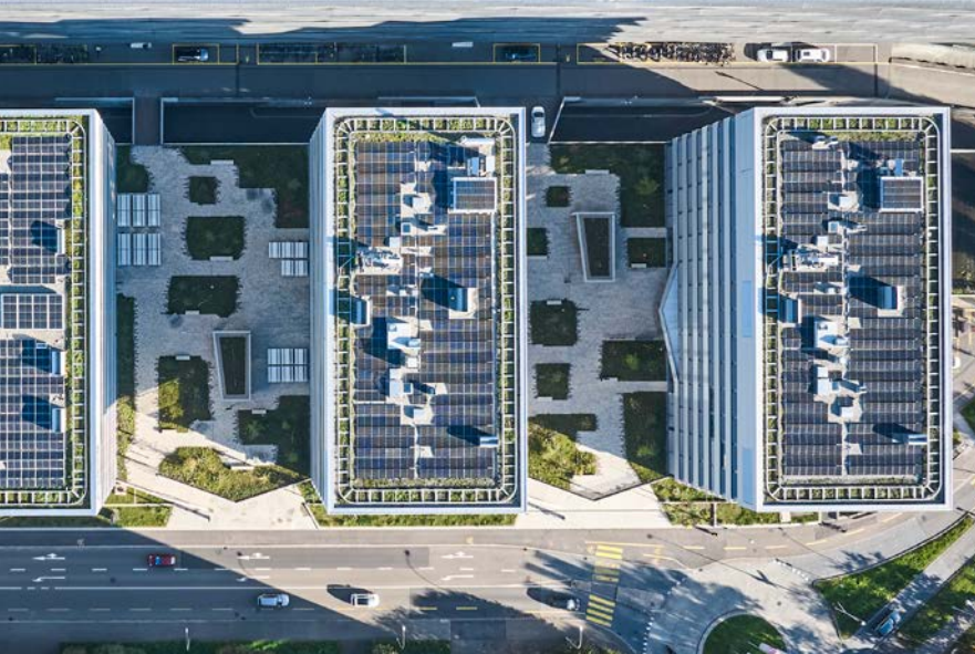
Photovoltaic system, Stücki Park Basel
