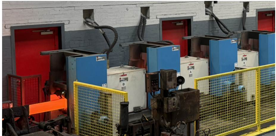
The new 12MW induction furnaces at Corby have reduced the site's direct emissions by 10%.
