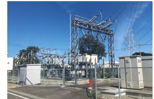
Okuma Switching Station
