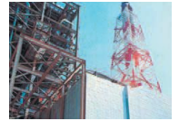
Denitrification equipment at Kudamatsu Unit 2
