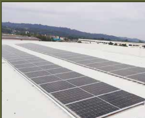
Solar panels at our Niella, Italy facility.
