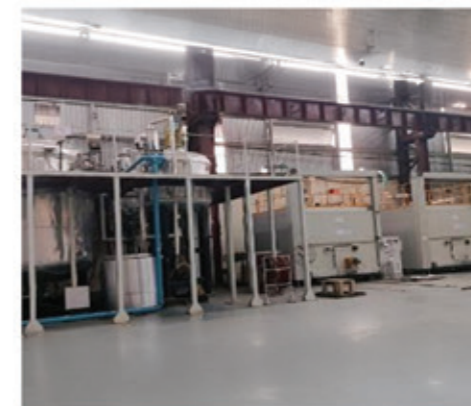
VPI Plant with Oven
