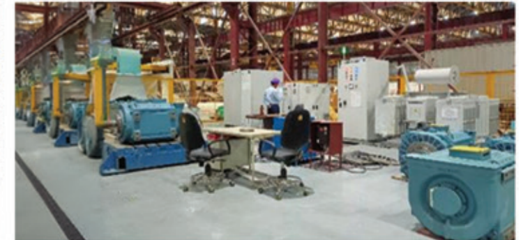
Traction Motor Testing Facility
