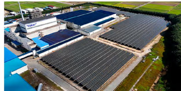
Ishikawa Plant Solar Power Generation Facility
