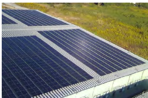
Solar power system
