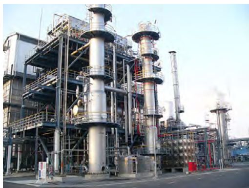
Isocyanate raw material production facility (CO plant)
