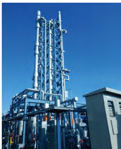
CO 2 Recovery PoC Trial Facility
