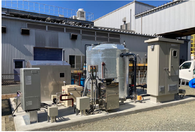
The food waste utilization system installed at our Toyohashi plant in fiscal 2023
