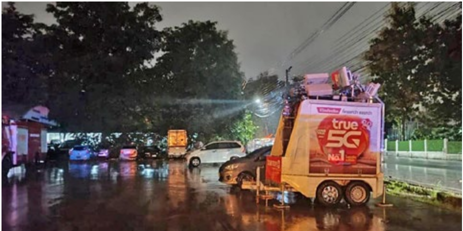
→ Prepared mobile Cell-on-Wheels (COW) units to support community and temporary accommodation areas
