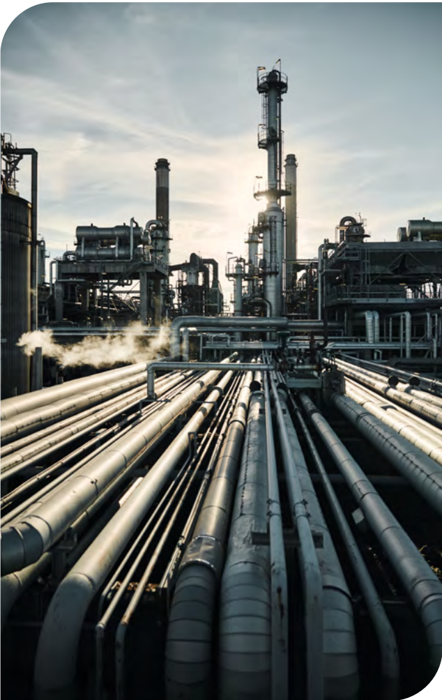
Processing units at the Gothenburg refinery in Sweden.
