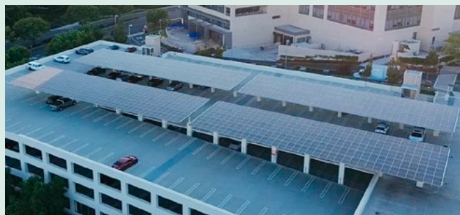
Newly installed solar power generation facilities (solar carports) (Left) MicroVention, Inc. (Right) Kofu Factory
