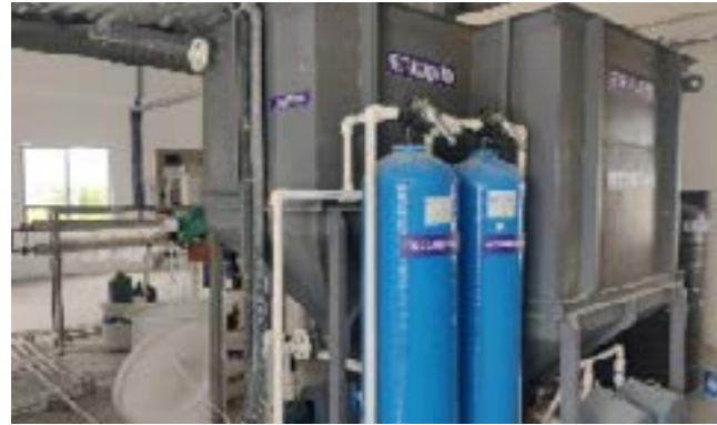
Domestic and Process water are recycled (STP & ETP with ZLD plant-100%)
