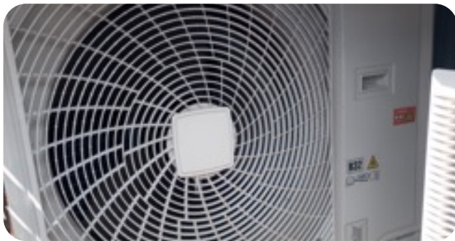
Lavender Lodge School Air source heat pump installed
