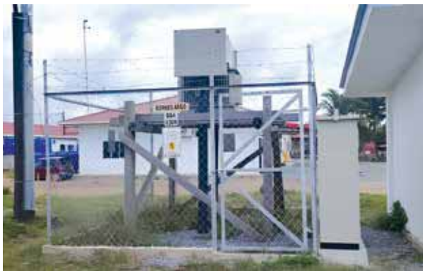
Sarawak Energy transformer at our plantation
