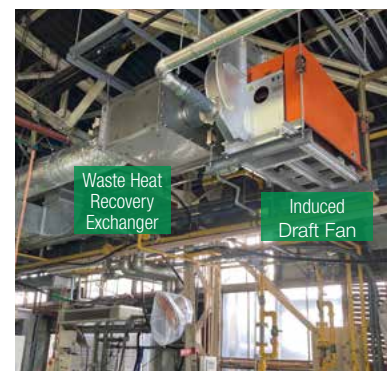
Heat Exchanger That Recovers Waste Heat
