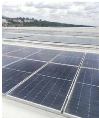
Solar Power System Installed at the Factory
