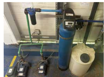
Treatment Tank and Filtration System
