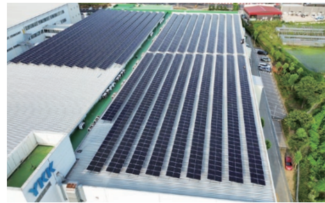
Solar power generation facilities (YKK Korea Co., Ltd.)
