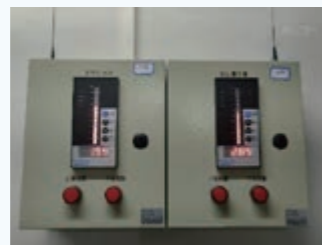
Water tank level gauges
