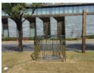
Underground rainwater collection tank
