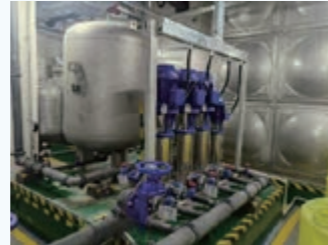
Landscaping water tanks and pumps
